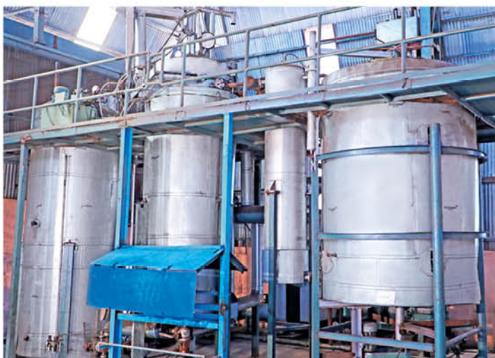
Pitch Impregnation Plant
